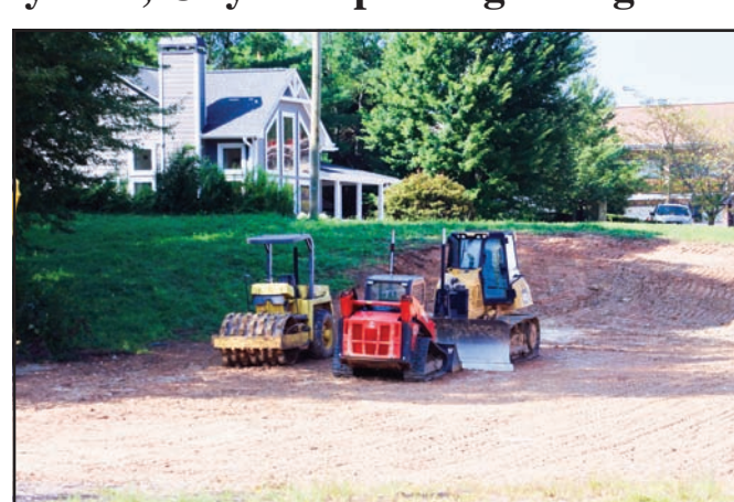
Site work began last week on the Arby's lot behind Blairsville City Hall. Photo by Shawn Jarrard
